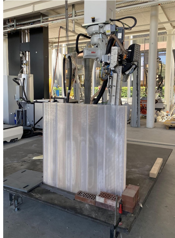
3DP façade sample fabricated at the Robotic Fabrication Lab in ETH Zürich
